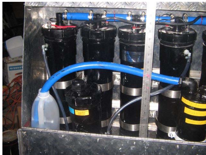
An example of housings for boosters
